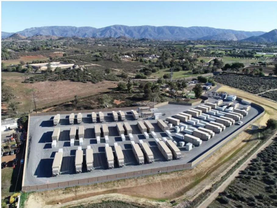
Terra-Gen’s Valley Center battery storage project opened in February 2022. A fire at the facility in September briefly shut down operations. (Terra-Gen)
